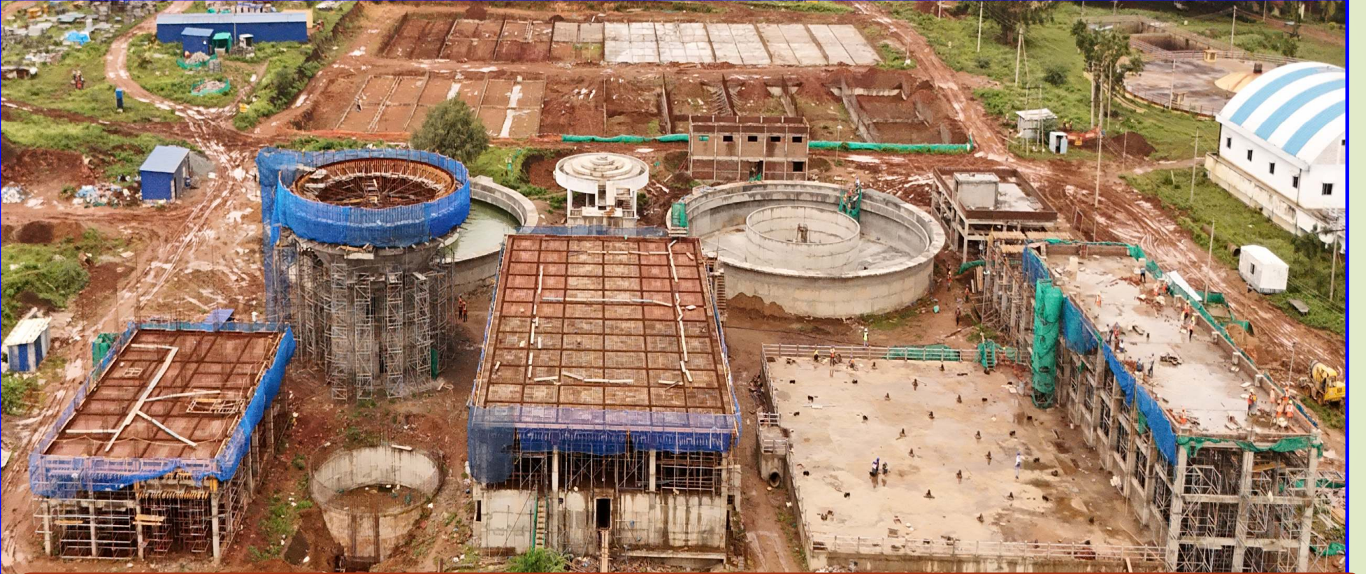
43 MLD Water treatment Plant
